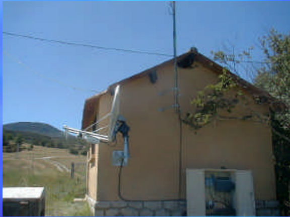
Trigance (Haut Var) Parabole, Coffret, Antenne Omnidirectionnelle, 14 Clients
